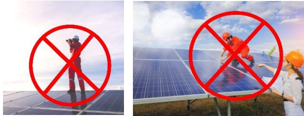
Image.1: Incorrect method of installation
